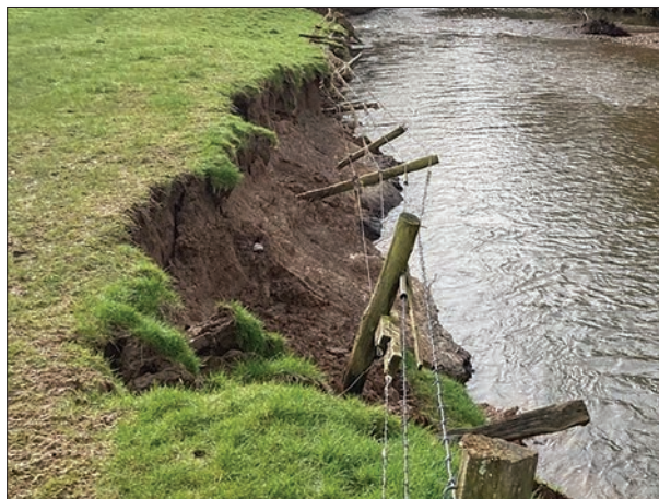
Riverbank before restoration
